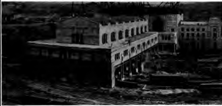
Union Station, Kansas City, Mo., (under construction) 1,000,000 square feet Sarco No. 6 Waterproofing.
